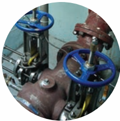
Waste Water Meter
